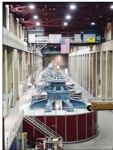
Main electrical transformers within one of the two powerhouses of Hoover Dam. [Source: Author, Ethan Chang]
